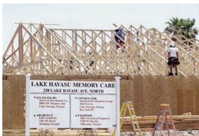
L.J. Frink/News-Herald Photo (Memory Care Center Photo) Construction workers are hard at work in this July 22 photo, helping to build the new Lake View Terrace Memory Care Residence that is located at 320 N. Lake Havasu Ave. and scheduled to open February 2009.
